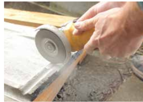
Grind a slot in the tile using an angle grinder with appropriate disc for example a diamond tip or masonry grinding disc.
