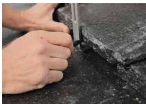
Place the tile where it will sit and mark out the size and position of the slot.
