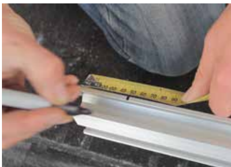
Mark the top of the rails where the edge of the panel will sit, this is typically 50mm in from the ends.
