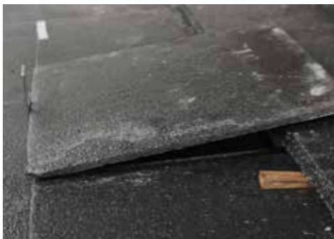
When replacing the removed tile where the bracket is positioned a slot should be ground to accommodate the thickness of the bracket and allow the tile to sit flush with the surrounding tiles.
