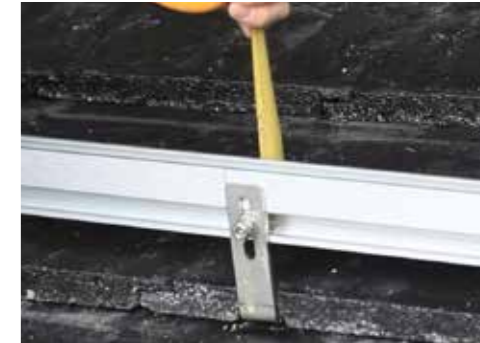
Set the height for your rail to sit - ideally the top of the rail should be 100mm to the top of the tile.
