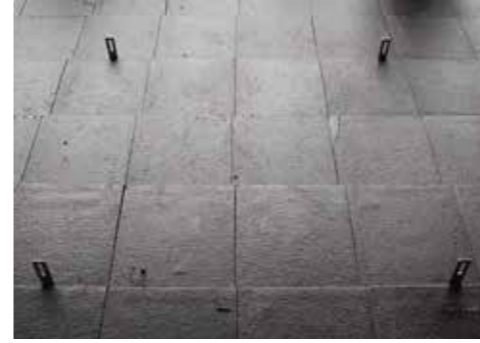
Once your brackets are installed you are ready to mount your rail to the Solar Adjustable Tile Brackets.
