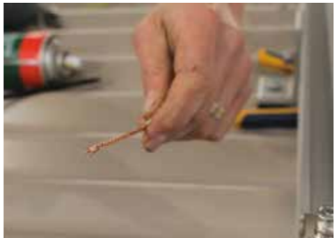
Use 4mm earth bonding wire and strip section of wire using wire strippers. Twist cable tightly.
